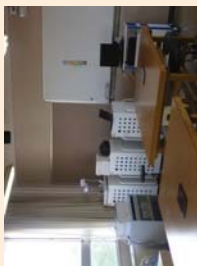
ICT installation in the laboratory classroom of applied physics
